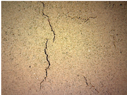
Shrinkage cracking at high layer thickness: 0-sample
